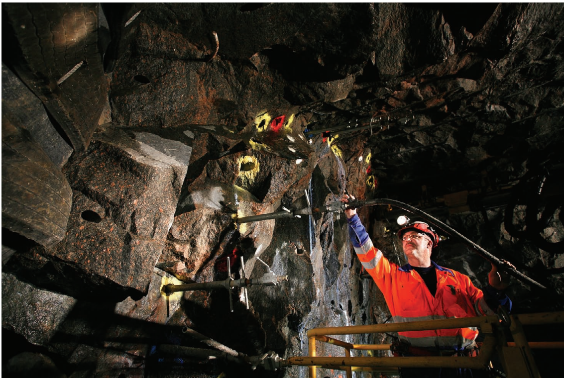
Figure 4-1. Checking of the equipment at the tunnel front in the experiment Sealing of Tunnel at Great Depth (photo: Curt-Robert Lindqvist).
